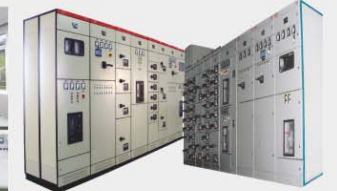
Series of electrical controlled equipment area
